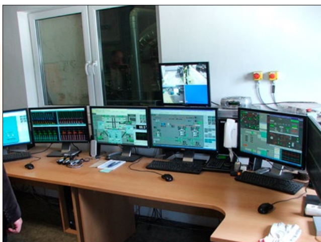
Figure 1: Controll system of power plant Bučina
